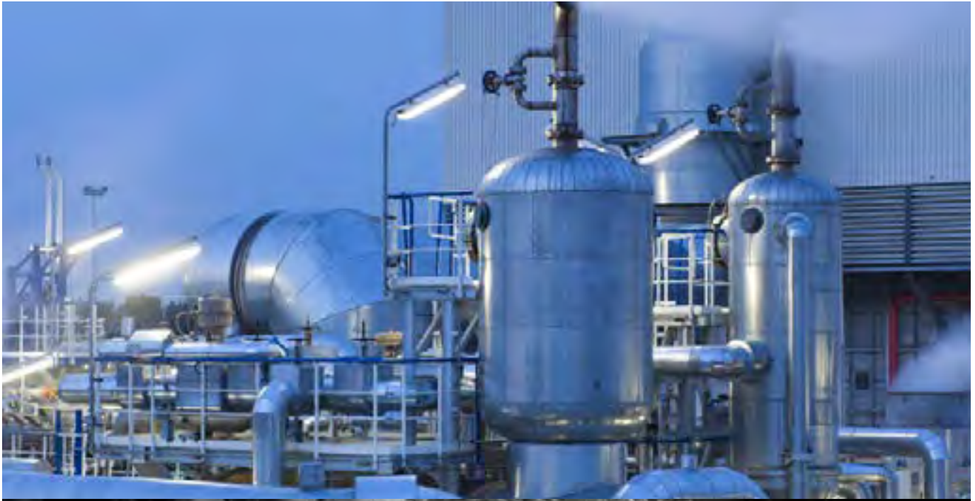
Producing hydrogen through steam methane reforming (SMR). Photo courtesy Air Liquide Engineering & Construction.
