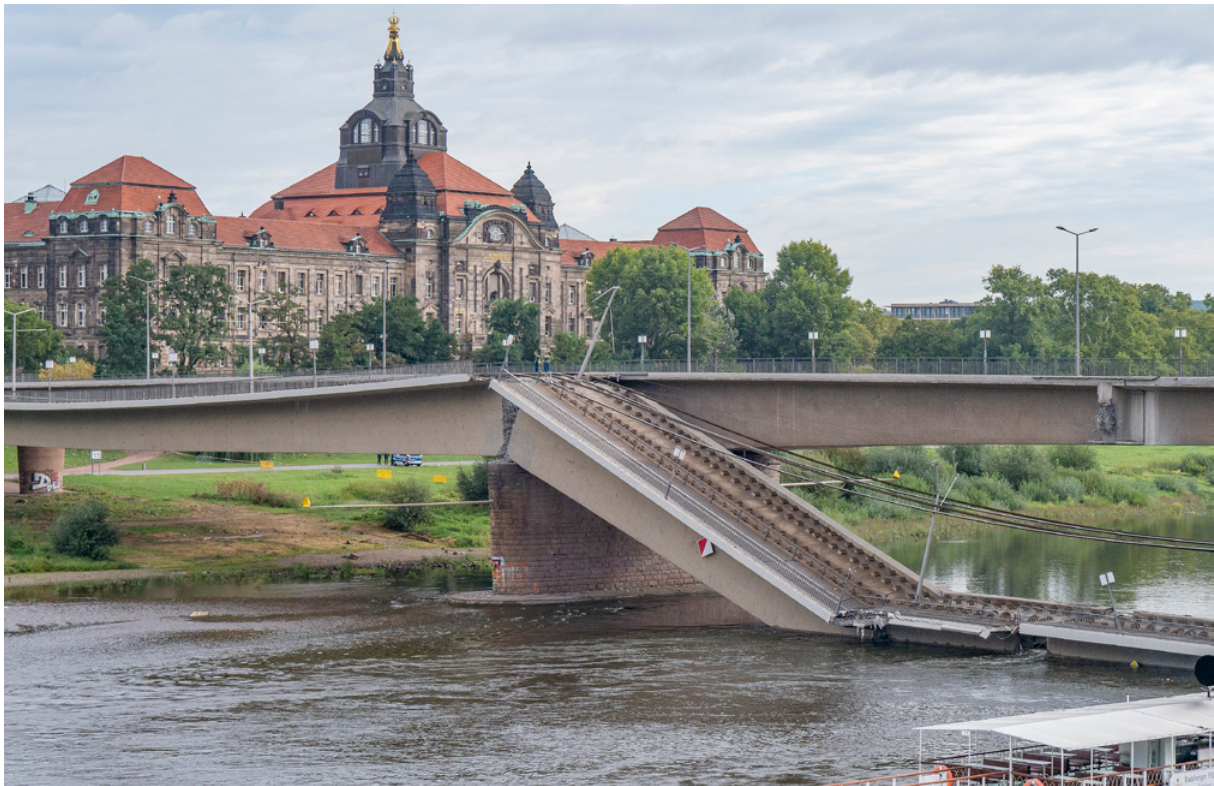
Figure 2.13: The Carolabrücke in Dresden, Germany, after a sudden collapse in 2024.
